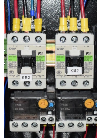
Figure 5-3: Vacuum Pump Contactor(s) with electrical wires and ground attached
