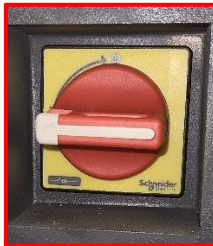
Main Power Isolation Switch
